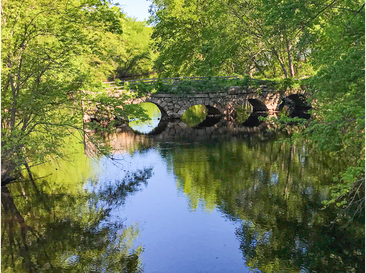
Current day view of Stone's Bridge facing north, downstream, from Stonebridge Road.
